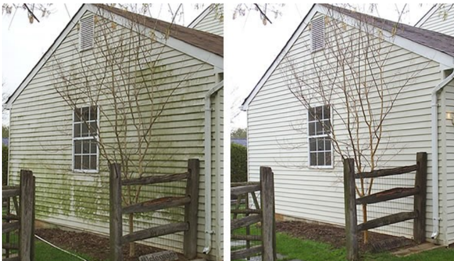
Above: Failure to meet the standard.
